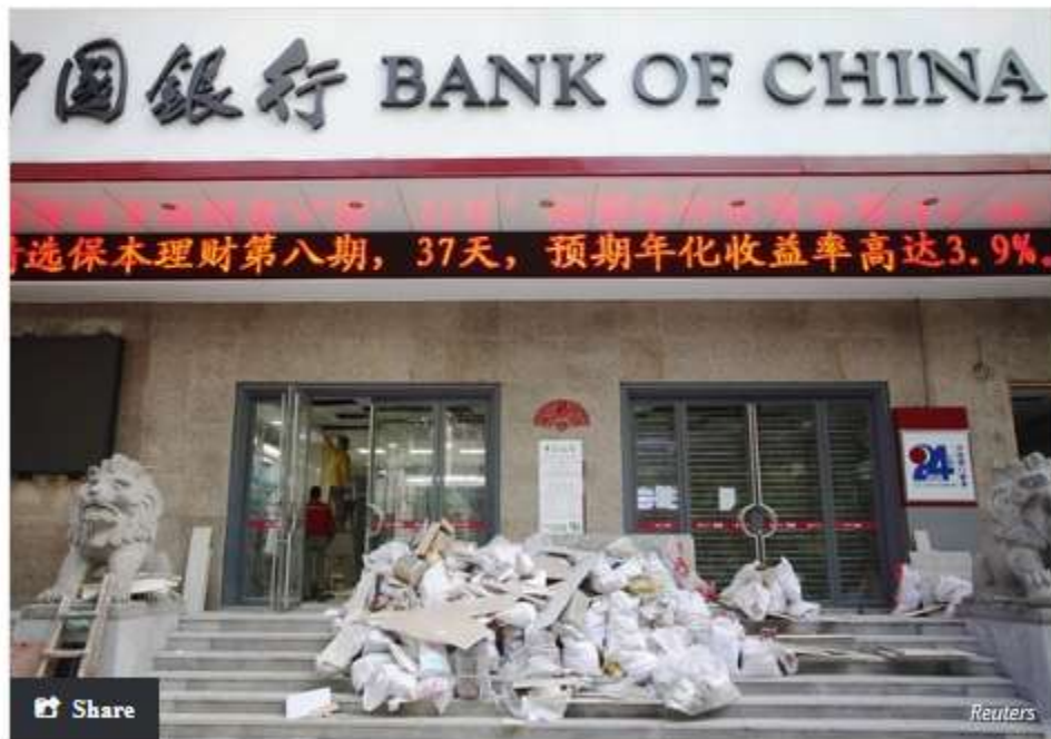
A Bank of China branch under construction early this year in Guangzhou, Guangdong Province.
