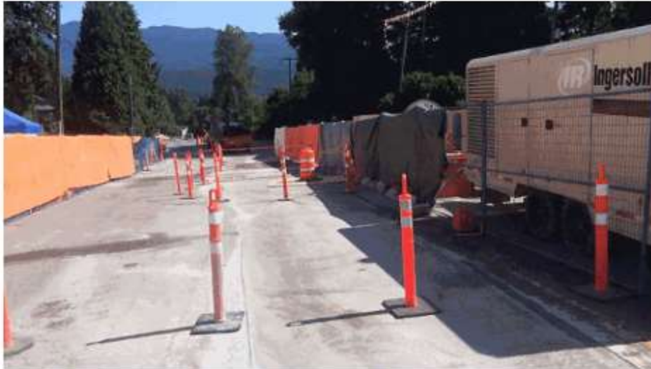
The sinkhole has been filled, but Clarke Road south of Seaview Drive is still closed to traffic.
