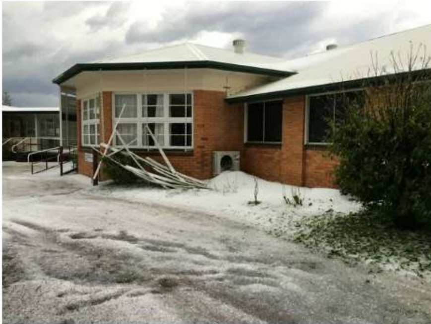
A hailstorm caused severe damage to Chinchilla Hospital.
