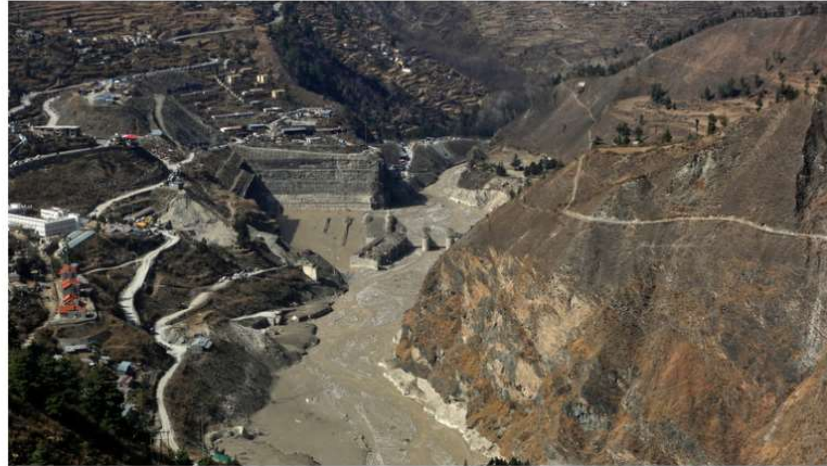
An aerial view shows a damaged barrage after a flash flood swept a mountain valley destroying dams and bridges, in Tapovan in the northern state of Uttarakhand, India, (FILE PHOTO) © REUTERS/Anushree Fadnavis
